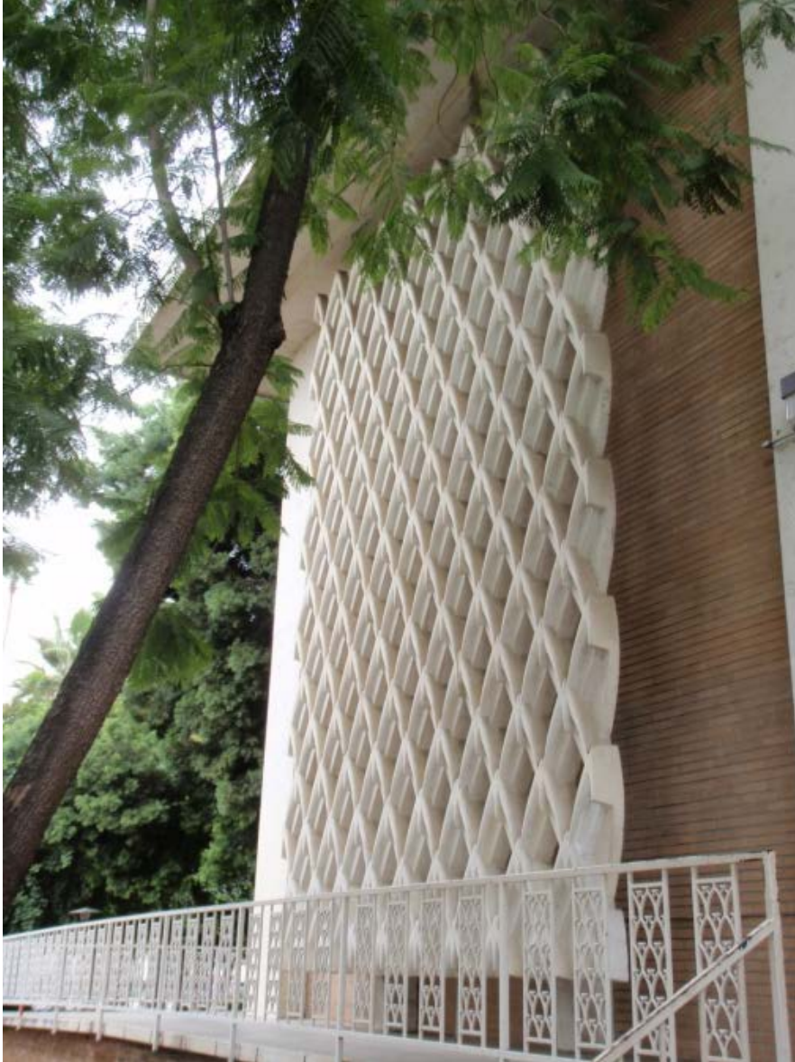
Figure 4 Riverside Main Library, detail, latticework screen. Also shows non-original handrail slated for removal. Source: Page & Turnbull, December 2011.
