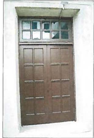
E HISTORIC COURT DOORS
