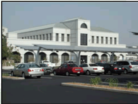
This carport is covered in solar panels, providing shade while producing clean energy.
